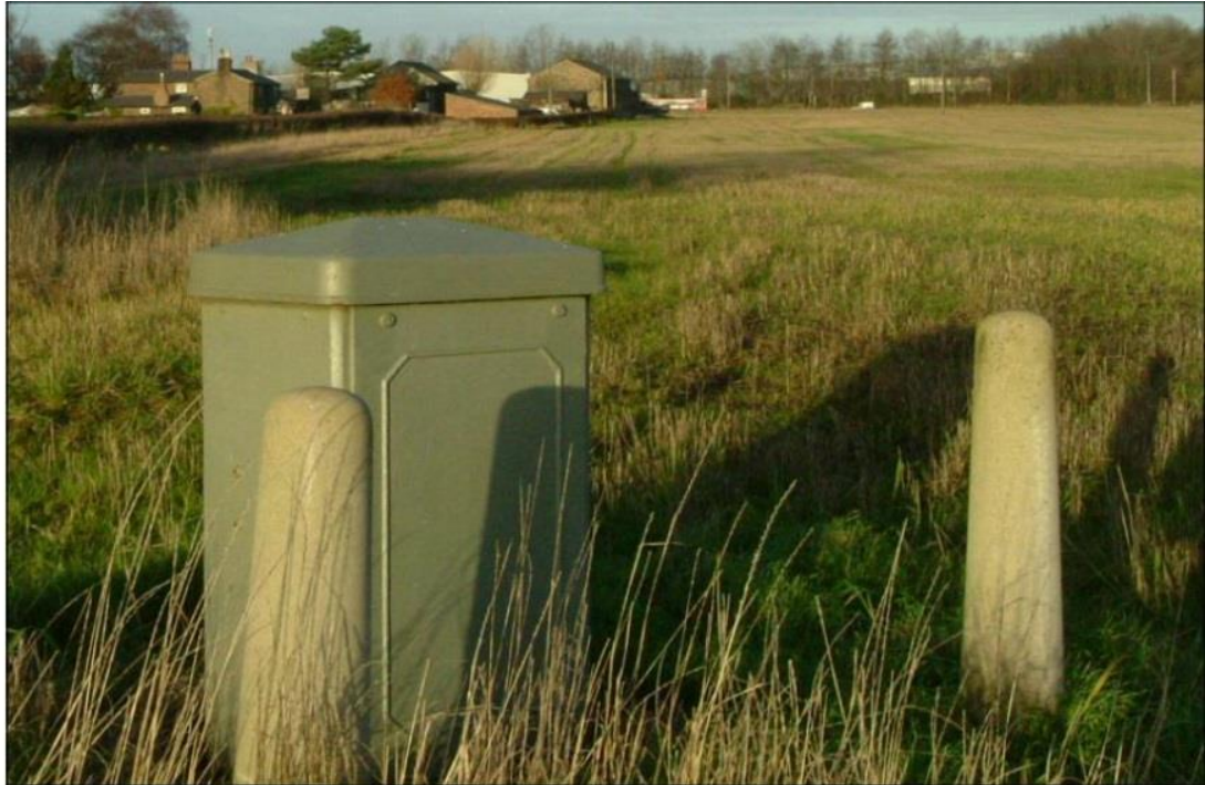
Figure 10: Photograph of Above Ground Inspection Kiosks for UGC
