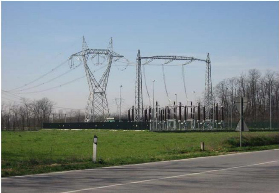
Figure 11: Example of a 400 kV Underground Cable to Overhead Line Transition Station
